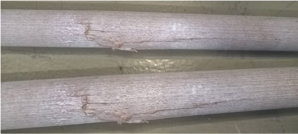
Figure 81 - Bar 5: cracked veneer
