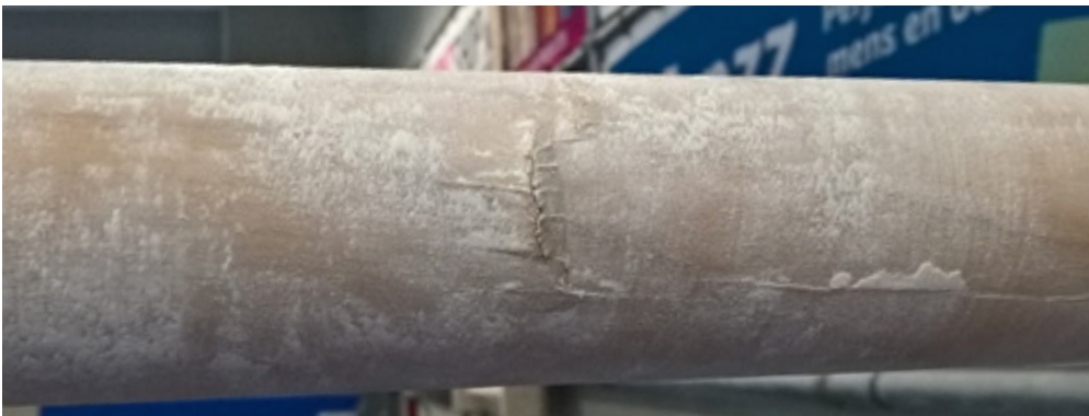
Figure 59 - Vertical crack after an hour of routines. The crack is bends outwards, creating a bump.
