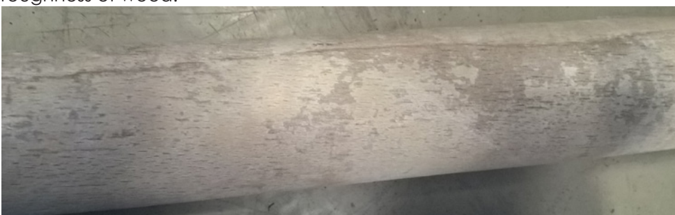
Figure 75 - Bar 3: abrasive wear
