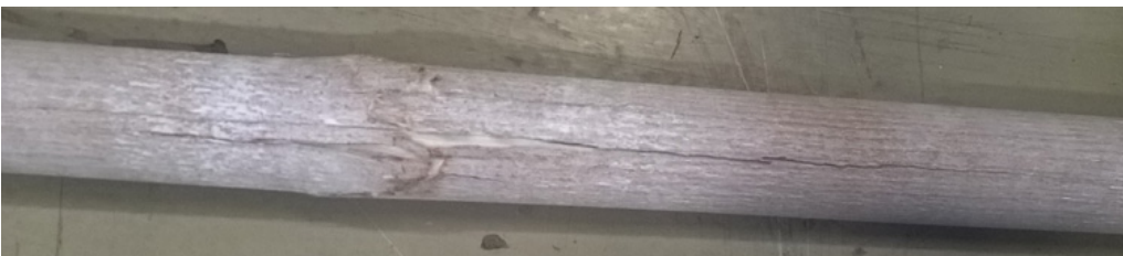
Figure 79 - Bar 5: Cracked veneer
