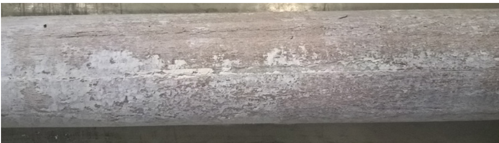
Figure 104 - Bar 9: worn patches at seam
